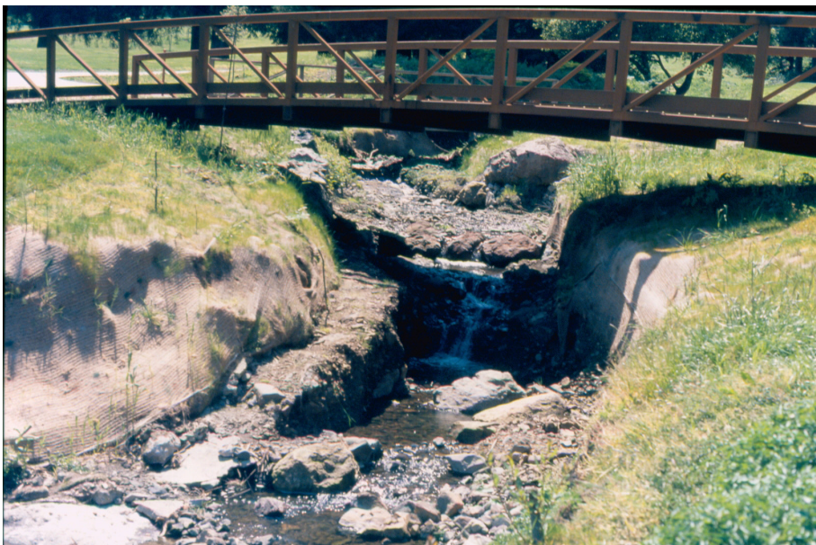
Photo 3: Headcut erosion in stream bed
