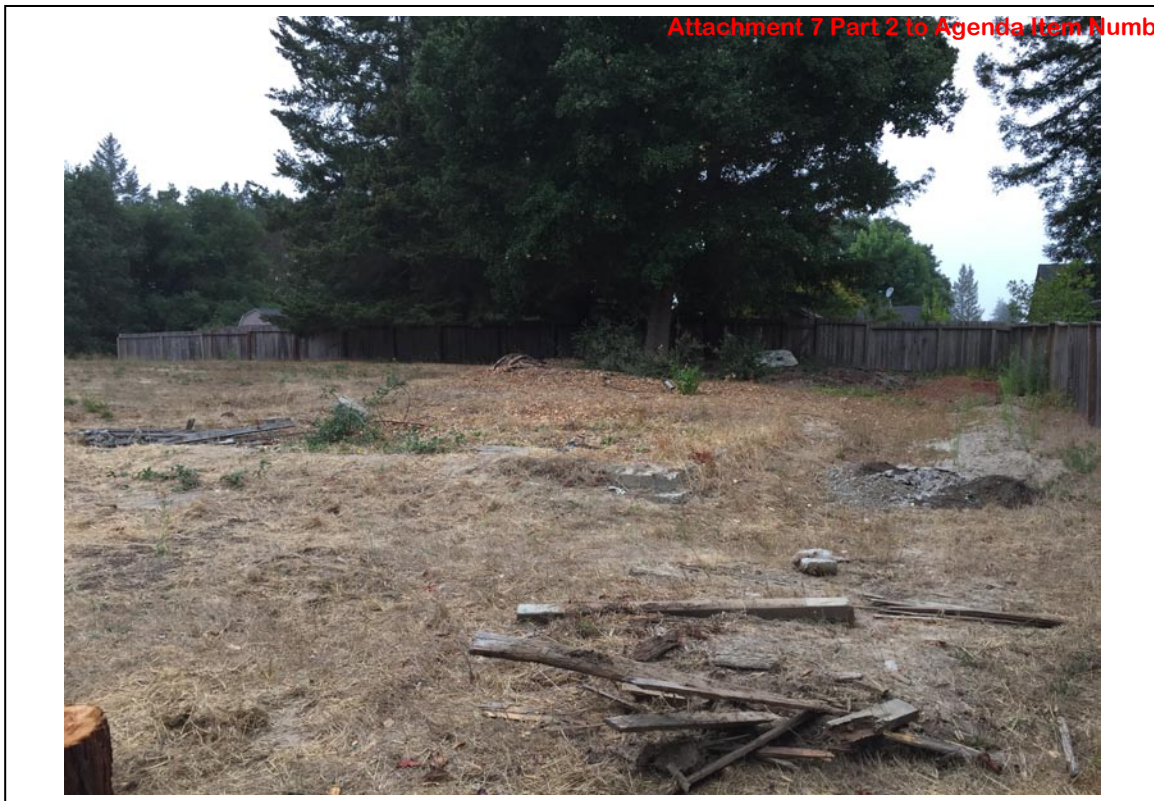
Photo 5: View from northeastern boundary of property looking west at construction debris and soil piles north of concrete slab.
