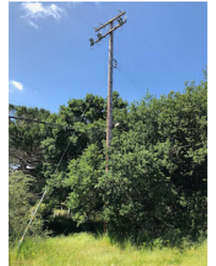
18 Power pole @ front of site
